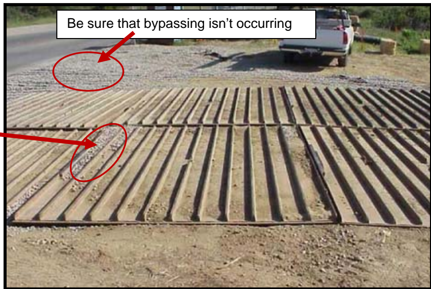
Manufactured metal plates knock dirt off vehicles before exiting a site.
