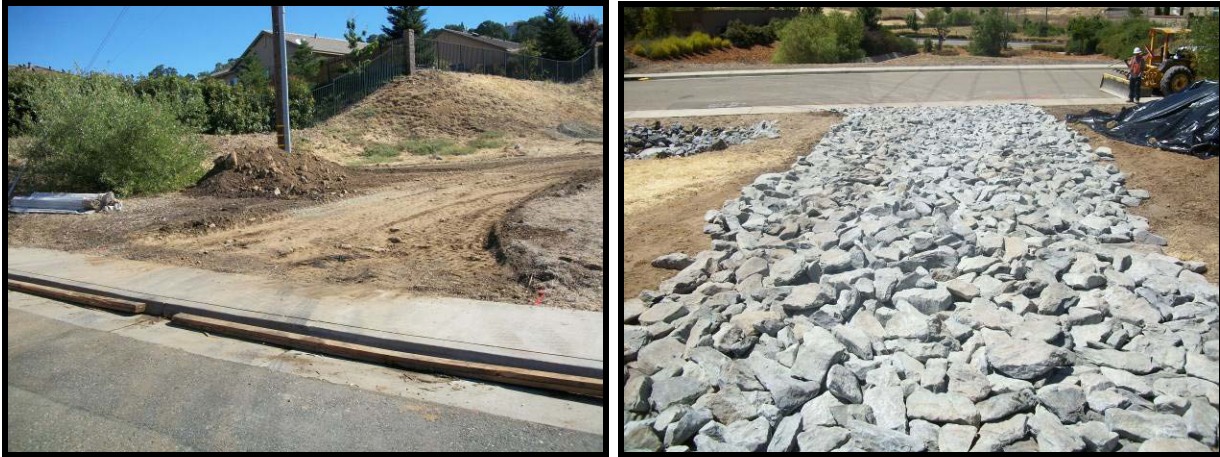
Construction entrance/exit before and after installation of gravel over geotextile fabric tracking control.
