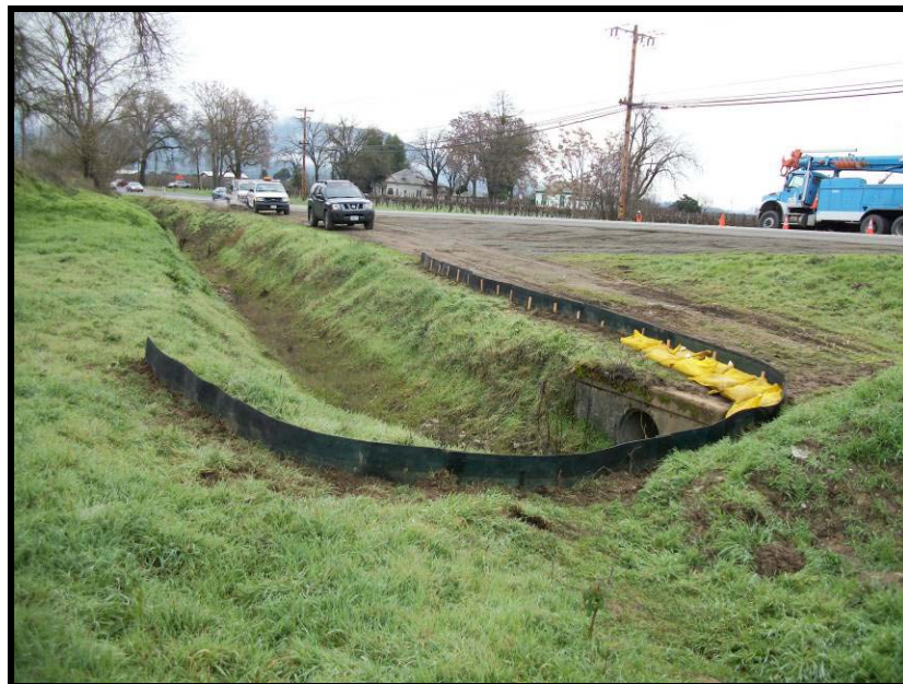
Silt fence reinforced with gravel bags, protecting a drainage channel.
