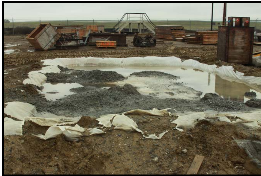
Adequate volume and maintenance are essential to prevent a release of high pH water from temporary concrete washout containments.
