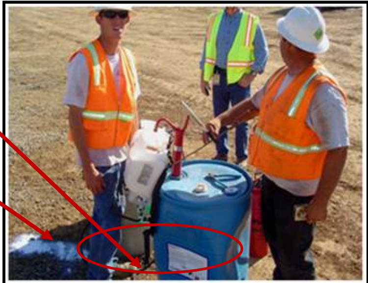
Example of improper use of materials. Missing secondary containment and spill kit.
