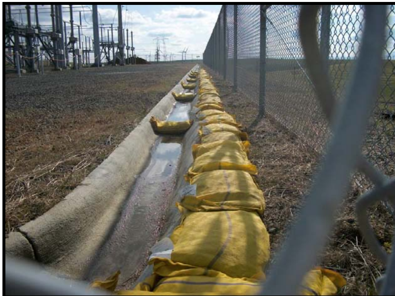
Gravel bags used to slow sheet flow run-on into the lined swale, and as check dams to slow flow within the swale.
