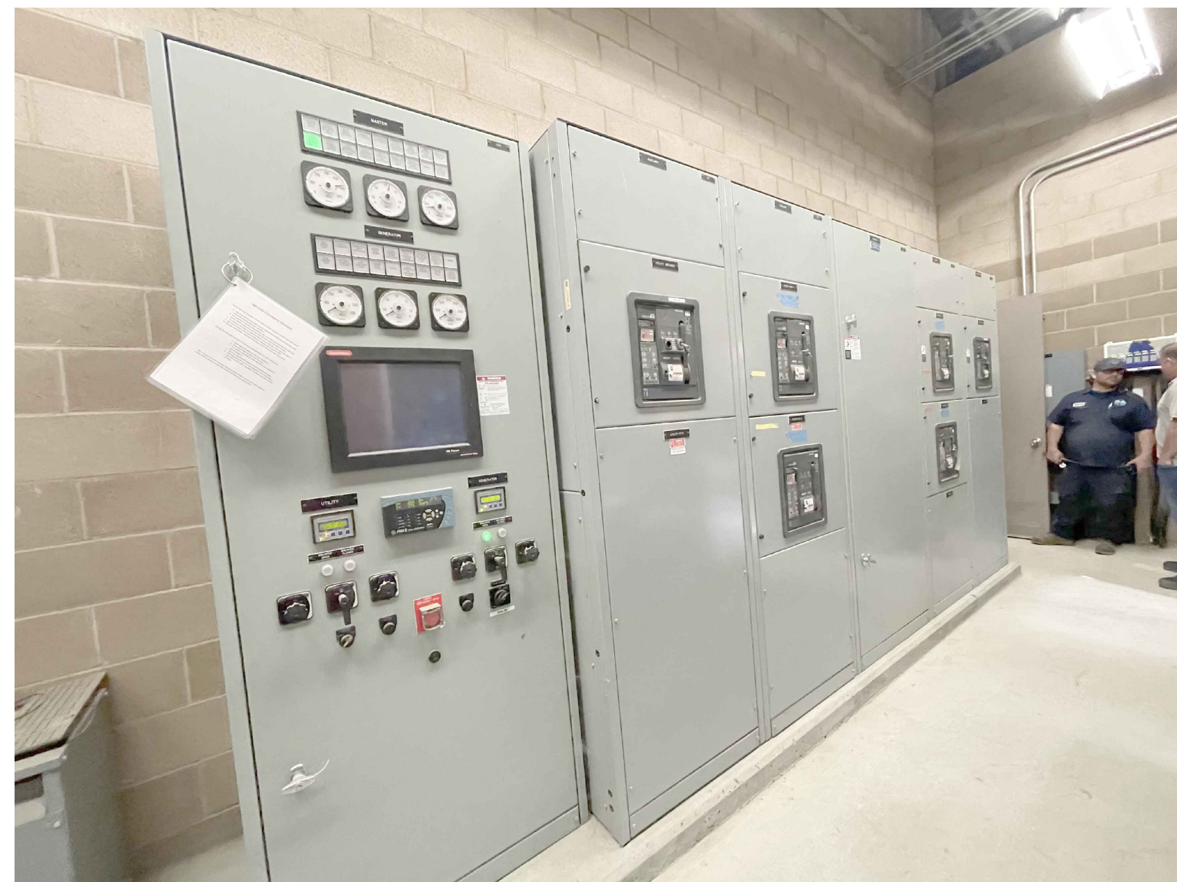
PEAK POWER SWITCHBOARD PHOTO 1 SCALE: NTS E480
