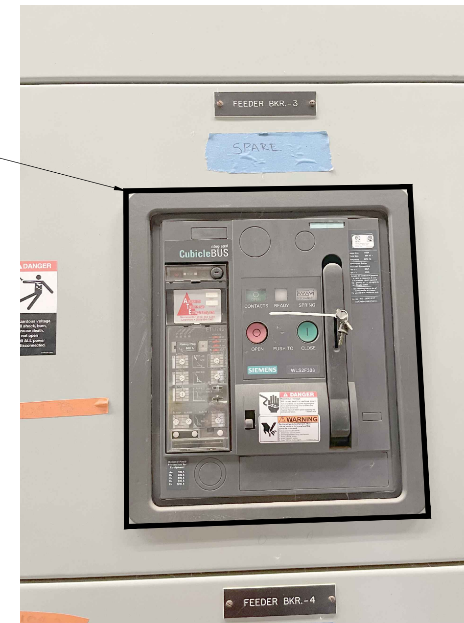
SPARE BREAKER TO BE REPLACED (MCC-30 BREAKER) PHOTO 3 SCALE: NTS E480
