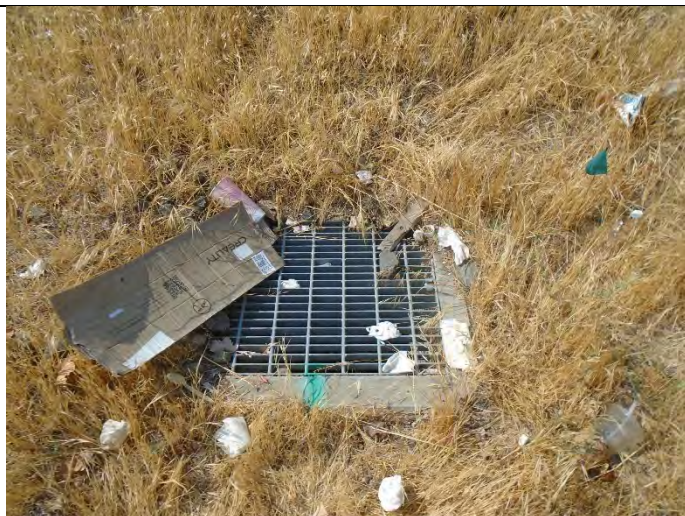
View North of onsite storm drain in southern portion of Property
